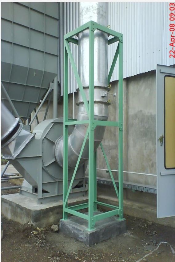
Construction Duct for Stack Dedusting Equipment
